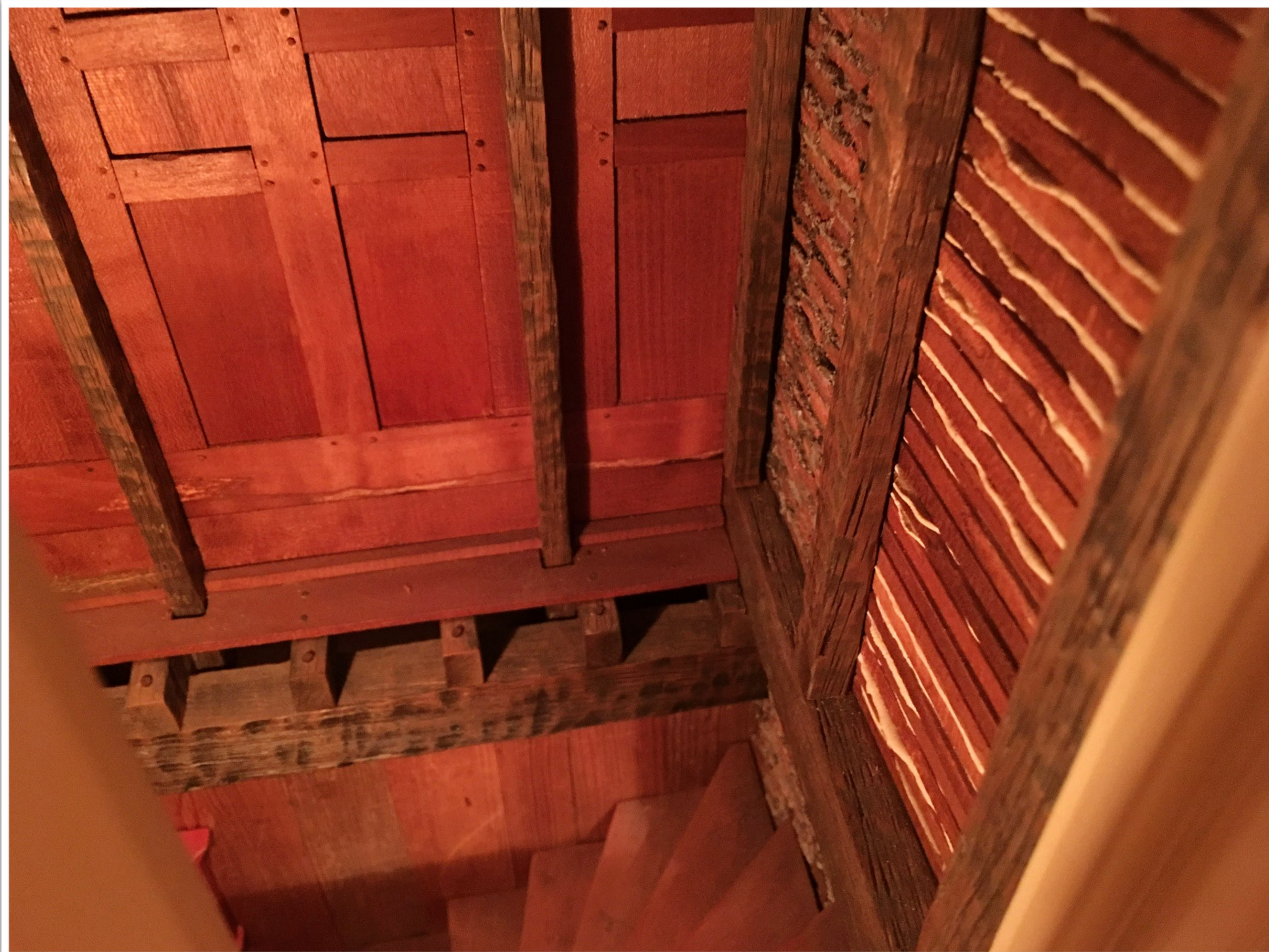
Back Stairs featuring hand hewn beams, pegged paneling. back side of plaster and brick
